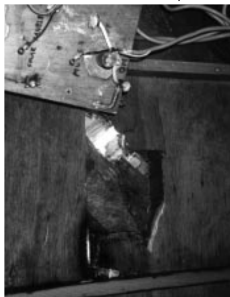
Aft hole inside. Darkened area is moisture, not char. Planking buckled inward.
