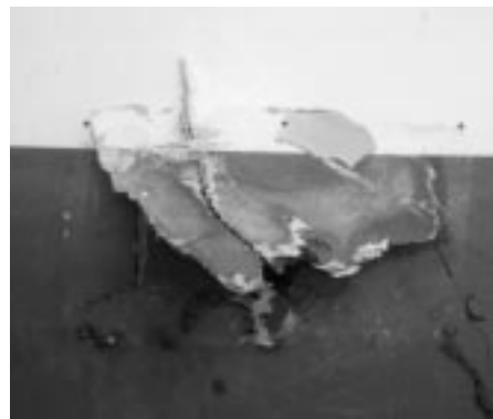
Aft hole outside. Fiberglass sheathing buckled outward.
